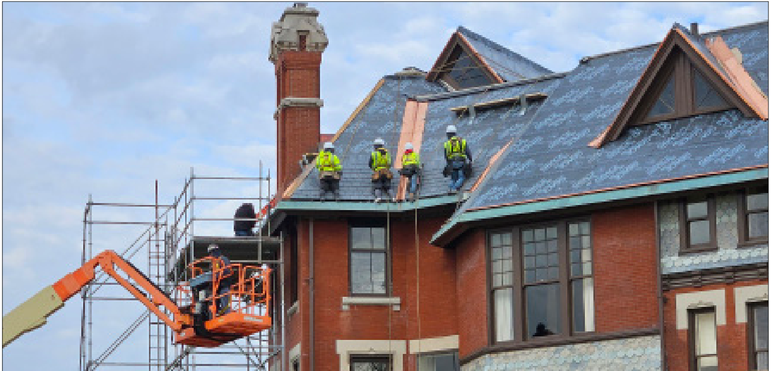
The mansion slate roof required a full replacement in 2023 following damage resulting from the 2020 derecho. This work had been delayed due to contractor and material availability.
